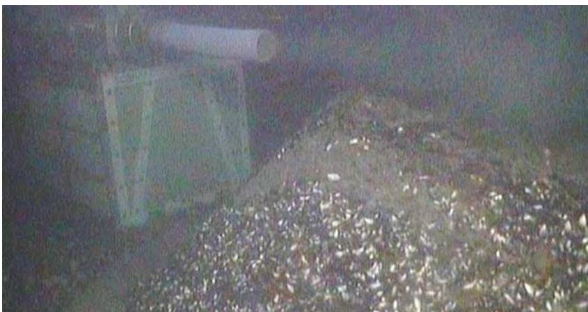
Figure 7-2. Photos of subsea suction dredging exhausts. Sediment/water plume at the top and middle, and a heap of settled materials (a significant volume of shells from mussels) at the bottom.
